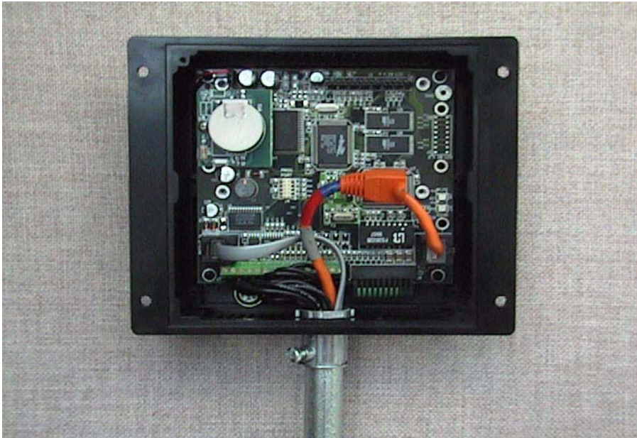
Figure B-10. Rear View of Intellicom with Outer Casing Showing Wiring from Conduit
