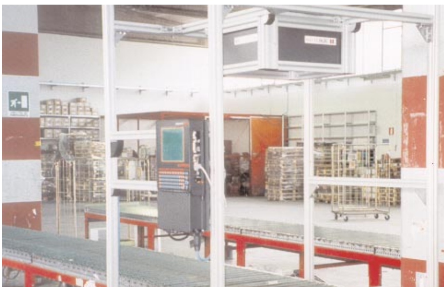
DS8100 omni-station in top side reading controlled by SC8000
